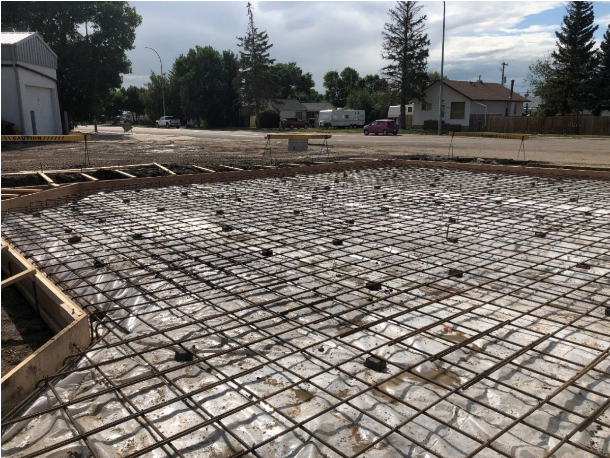
Formwork and rebar for concrete apron in front of new bay doors
