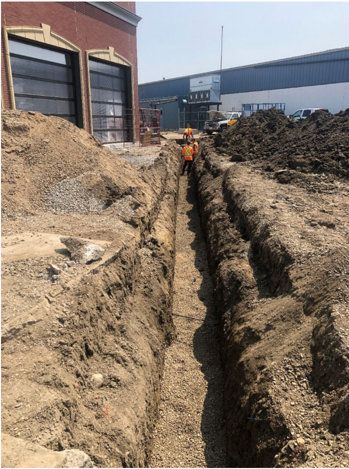
Installation of new storm branch line and catch basin in parking lot
