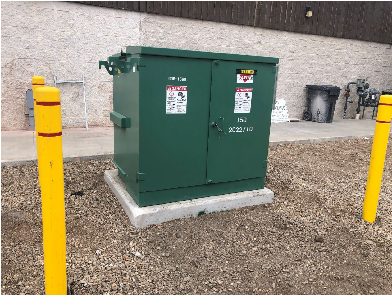
New 600-amp power service transformer installed by Fortis Alberta
