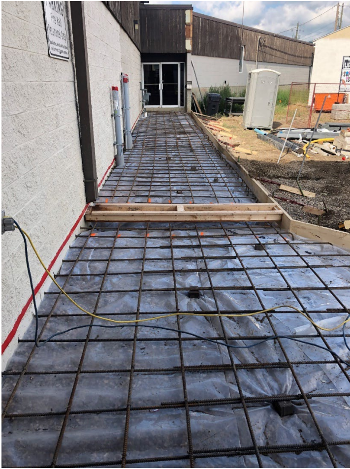
Formwork and rebar for exterior sidewalks on south side of existing building
