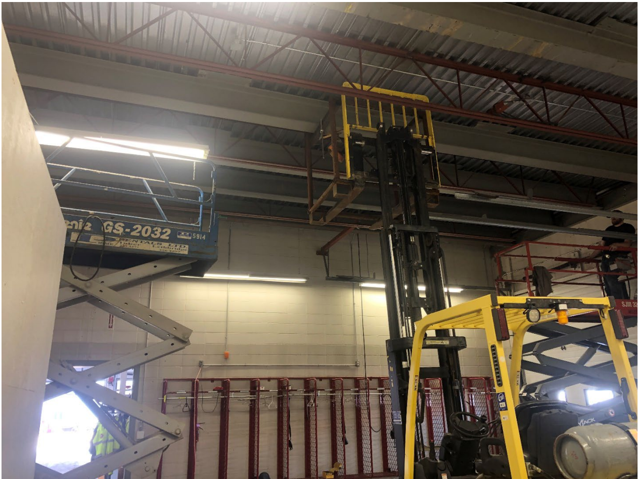
Installation of additional roof beams in existing bays to support snow loads from new roof
