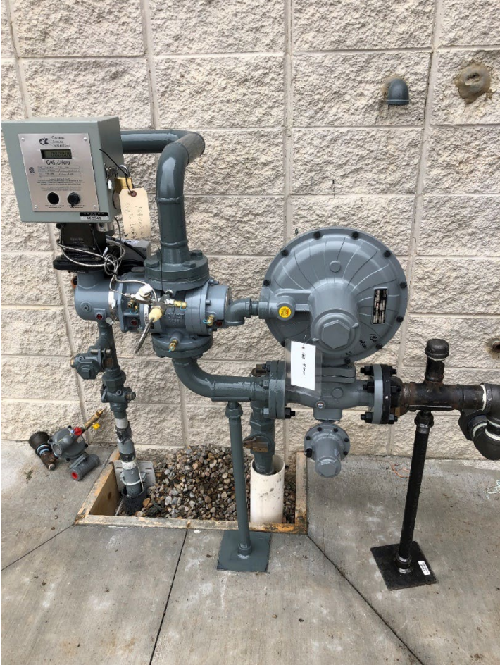
Upgraded gas meter installed by ATCO
