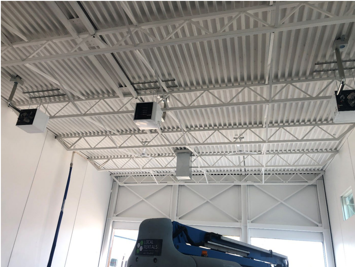
Interior HVAC equipment, 3 unit heaters, air makeup unit and 2 exhaust fans
