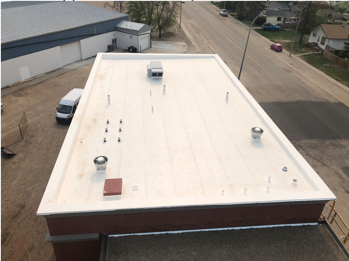
Aerial view of roof installation, air makeup unit and exhaust fans
